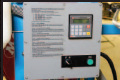
PLC (Programmable Logic Controller) control system.
